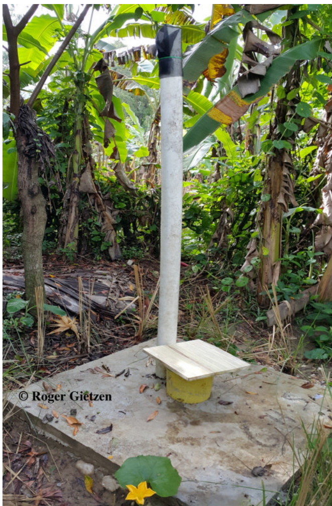
Ventilation pipe and a seat made of a plastic bucket. Notice the pipe is covered with mesh.
